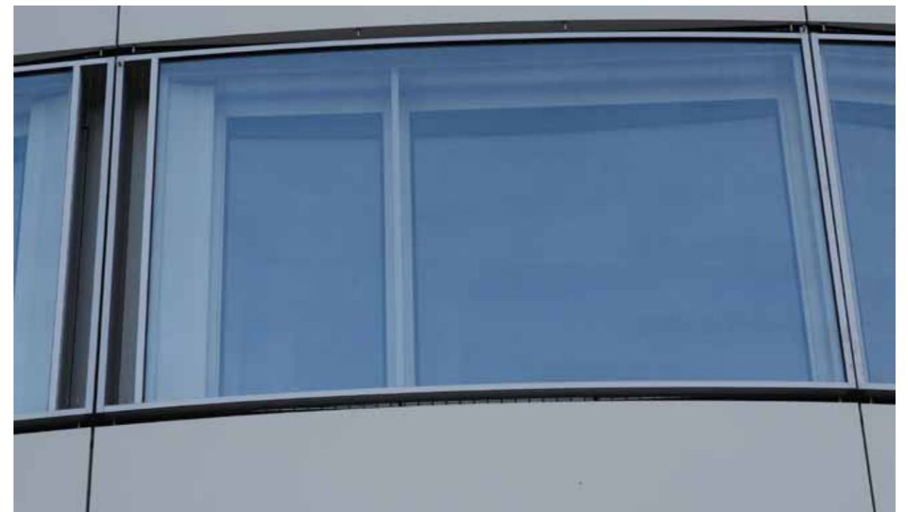
The outer shell of the new metal façade consists of curved sheets in which a flat fixed glazing sits. Their baffle discs are surrounded by inconspicuous shadow gaps with louvers.
